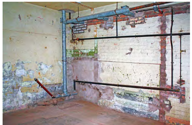
The former water tank room, in the control bunker in 2009. Evidence of modification to prepare it for its new role is clearly visible, including rerouting of pipework and bricking-up of the apertures to the adjoining room. The pipe visible at 45 degrees is where the post's toilet room will eventually be located. Photo Mike Norris
